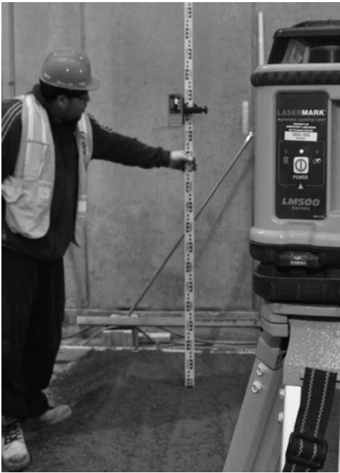
Used to check elevations of granular bases and to set formwork bulkheads to finished floor elevation
