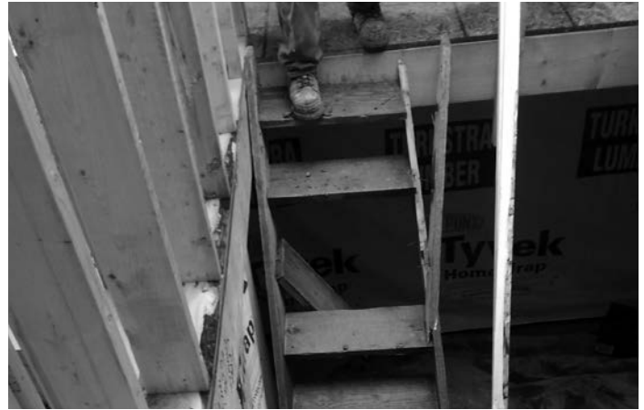
Figure 9-11: Stairway is too narrow and has steps missing
