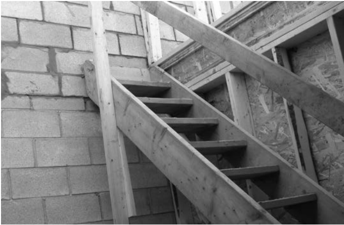
Figure 9-8: Stairway is poorly located
