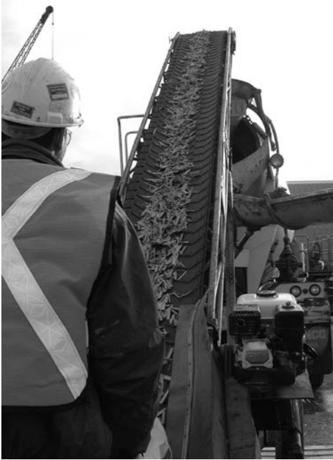
Used to install fibre reinforcing from the ground to the top of a concrete truck
